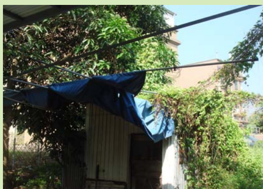
維修逢吉蔬菜產銷有限責任合作社構建物(前) Maintenance of Fung Kat Vegetable Marketing Co-operative Society, Ltd Building (Before)
