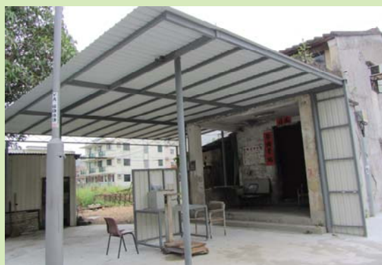
維修逢吉蔬菜產銷有限責任合作社構建物(後) Maintenance of Fung Kat Vegetable Marketing Co-operative Society, Ltd Building (After)
